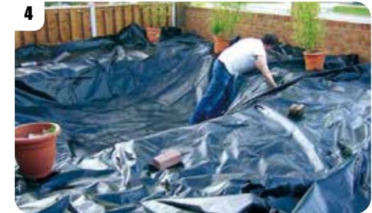
4 Once the liner has been unfolded it's time to smooth it into the shelves and corners as best you can (barefoot is best).
