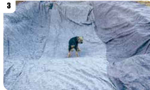
3 Due to the very stony nature of the ground we chose to upgrade to Fleece Underlay (Dog optional!)
